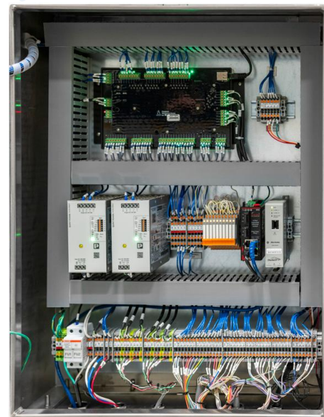
Gas Mitigation MICP™ Sub Panel
