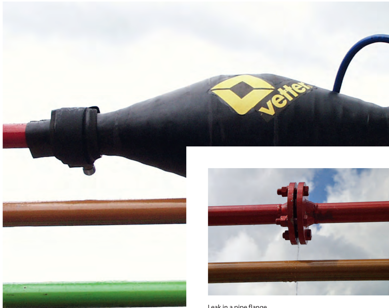
Leak in a pipe flange
