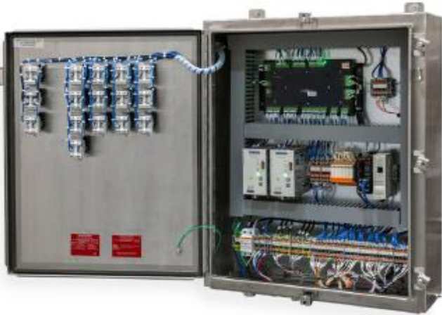
Gas Mitigation MICP™
