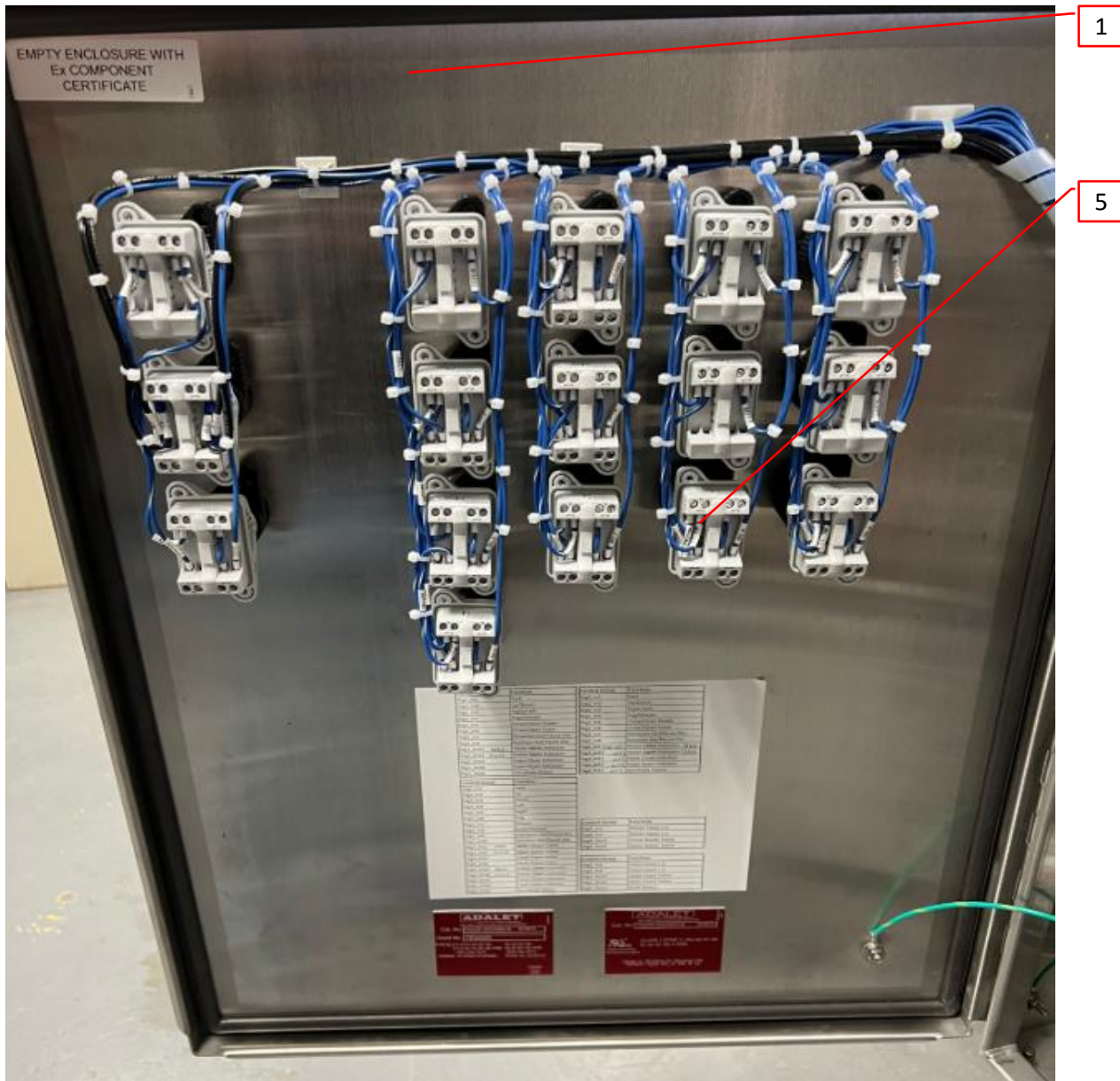
Photo 3 - Internal View of MICP Door
