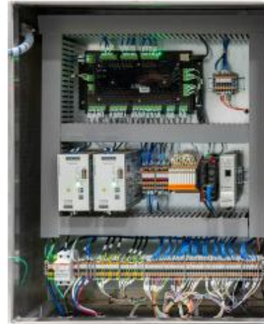
Gas Mitigation MICP™ Sub Panel
