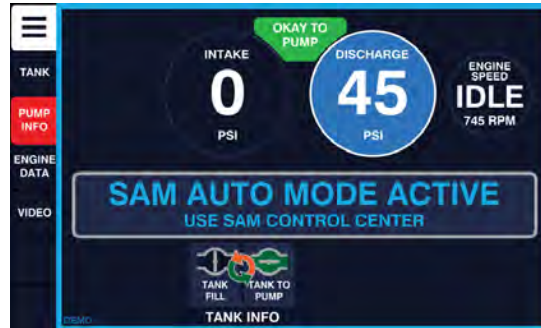
Figure 7. Pump Controller Tabs (Indicating Maintenance Required)
